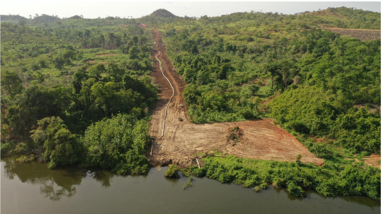
River Abstraction Area Clear, 90 KV Line Cleared and Pipe welding in process
